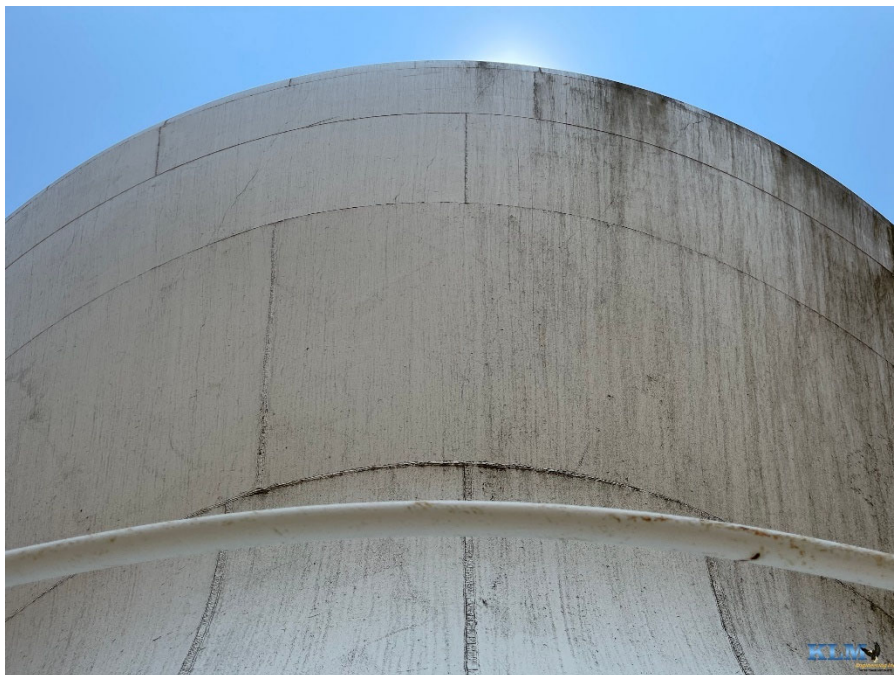
Photo No. 52 Condition of lower torus and bowl with painter's ring visible
