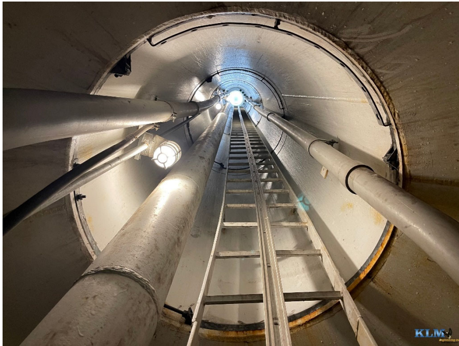
Photo No. 29 View of drywell tube
