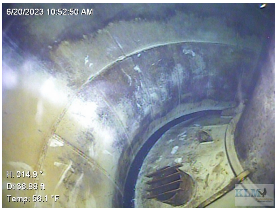
Photo No. 23 Bowl coating conditions with fill pipe visible
