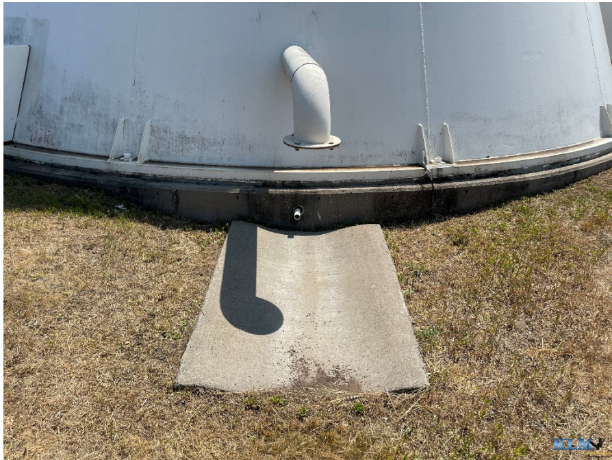
Photo No. 59 Overflow pipe outlet and splash pad
