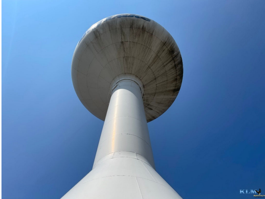
Photo No. 55 View of bowl, pedestal, and base cone
