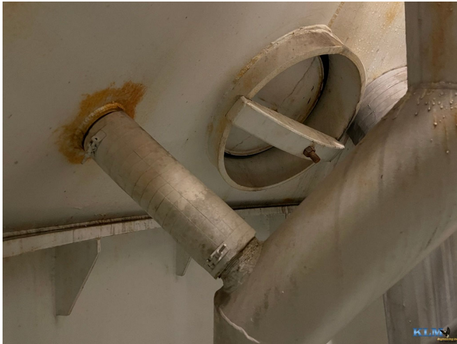
Photo No. 31 Bowl drain line and manway
