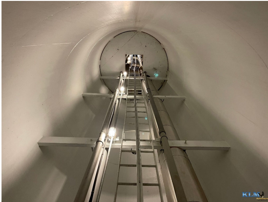
Photo No. 33 Pedestal conditions looking up at underside of top landing
