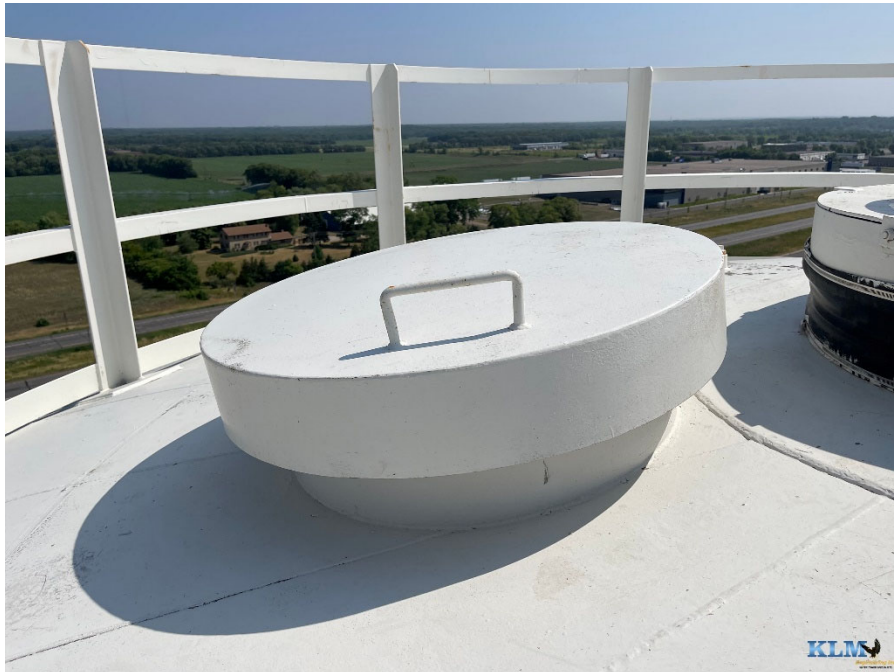
Photo No. 45 Wet access manway
