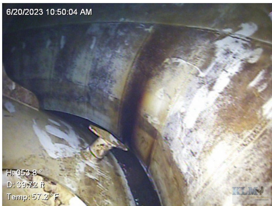
Photo No. 24 Bowl conditions with failures visible
